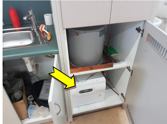
Photo 8. Interior, ground level, store kitchenette, hot water heater under sink – suspected SMF-containing internal insulation.
