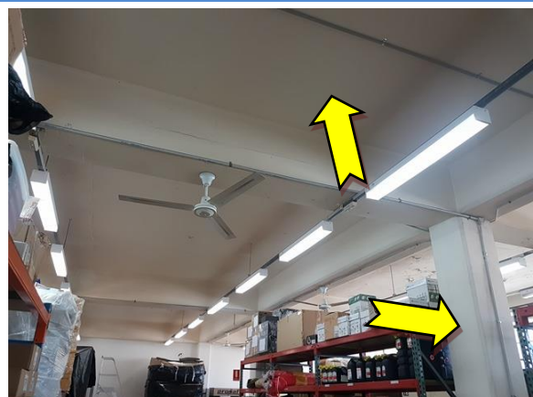
Photo 12. Interior, throughout, ceiling and walls – suspected lead containing upper white coloured paint system.
