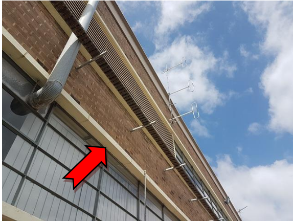
Photo 1. Exterior, throughout, eave lining – suspected asbestos containing fibre cement sheeting.
