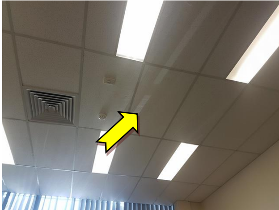
Photo 7. Interior, ground level, stores office, ceiling – suspected SMF-containing compressed ceiling tiles.
