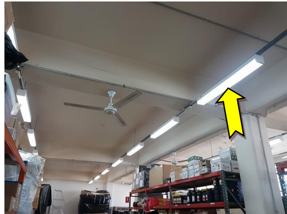
Photo 10. Interior, throughout, double tube fluorescent light fittings – suspected non PCB-containing capacitors.
