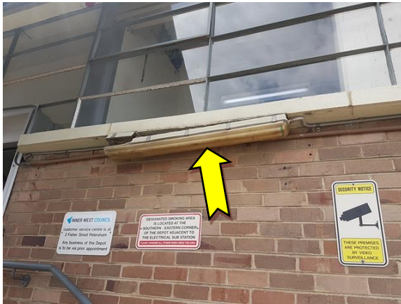
Photo 9. Exterior, throughout, single tube fluorescent light fittings – suspected PCB-containing capacitors.
