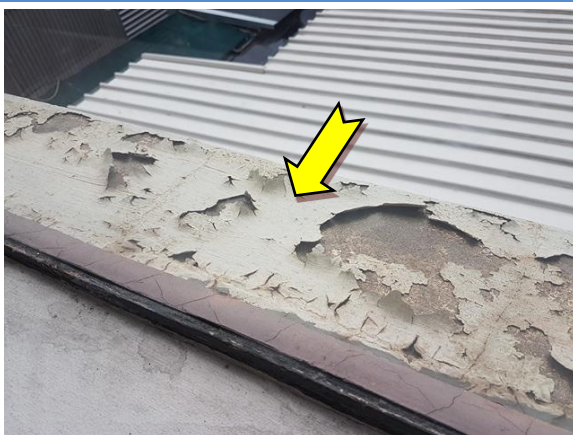
Photo 11. Exterior, throughout, window frames – suspected lead containing upper white coloured paint system.
