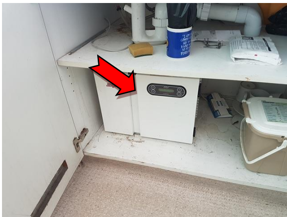
Photo 5. Interior, level 1, kitchen, hot water heater beneath sink – suspected SMF-containing internal insulation.
